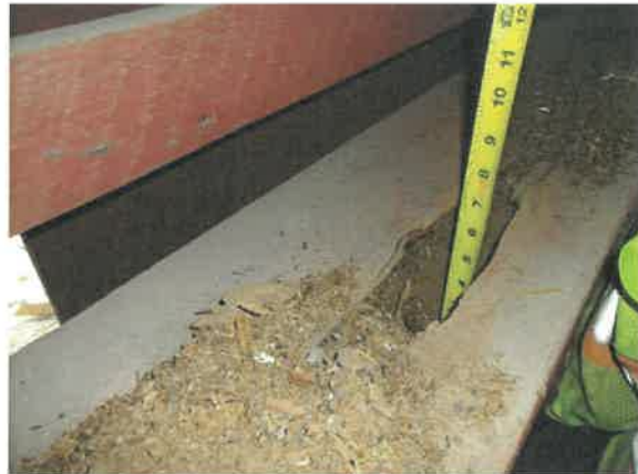
East Truss Top Chord Rot
