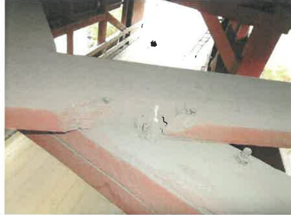
Broken Connection at Cross Beam and Diagonal
