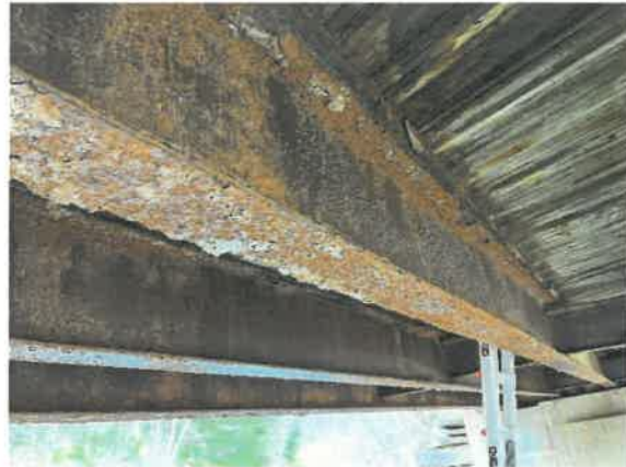
Interior Beam Rusting
