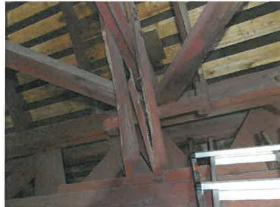
Broken Connection at Crossbeam and Knee Brace
