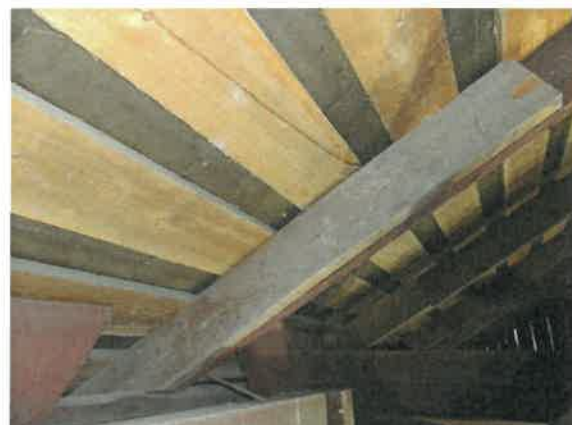
Split in Roofboard and Spliced Rafters
