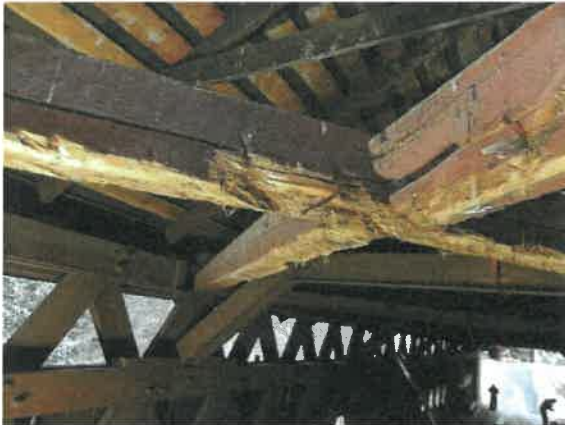
Impact Damage in Diagonal Bracing
