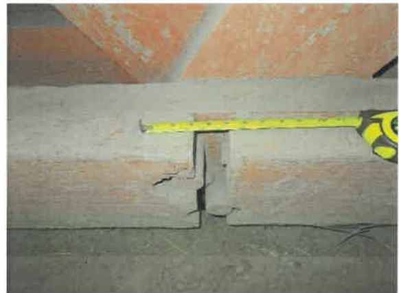
Gap in Chord 3 at Trunnels
