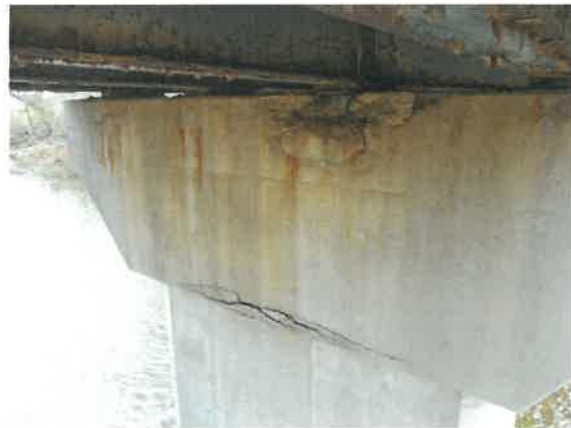
Concrete Spalling at Stringers Bearings
