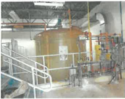
Caustic Storage Tank
