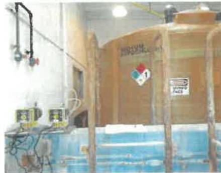
Sodium Hypochlorite Tank
