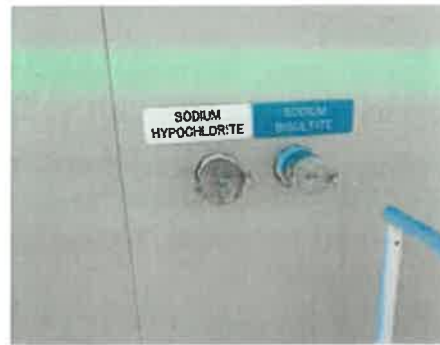
Truck Unloading Station
