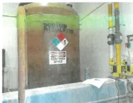
Sodium Bisulfite Tank and Pumps
