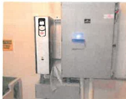
SBR Blower Control Panel
