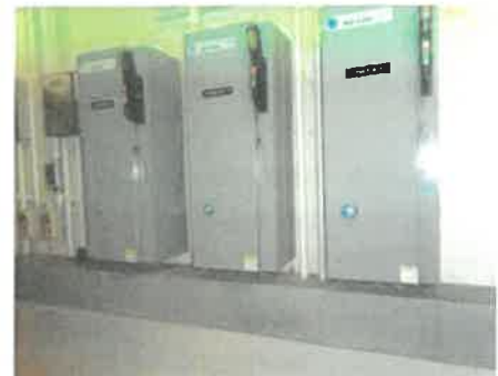
Sludge Conveyor Control Panels
