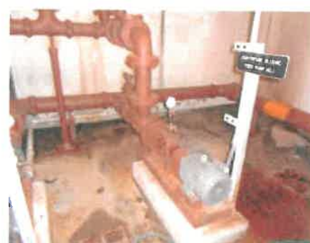
Centrifuge Sludge Feed Pump
