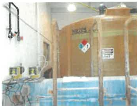
Sodium Hypochlorite Tank and Pumps
