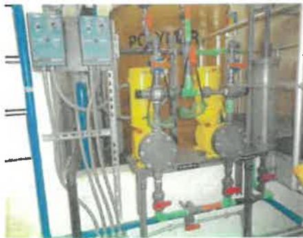
Polymer Storage and Pumps
