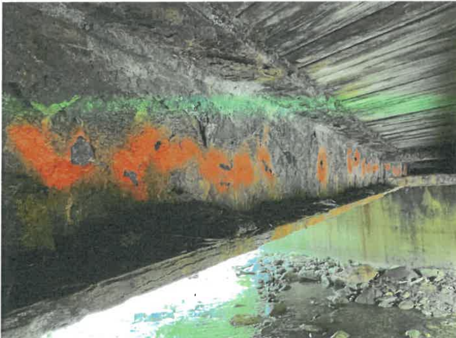
Stringer #5 – Numerous Holes in Web
