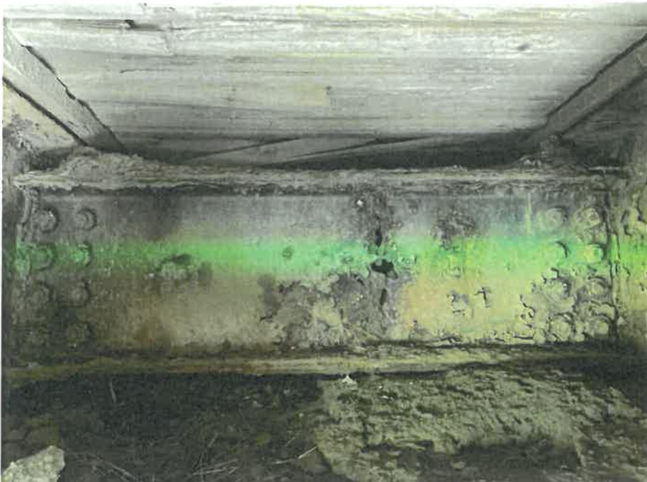
Deck Failure at Abutment #2 Between Beams #2 & #3
