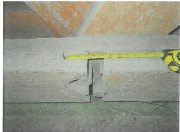
Gap in Chord 3 at Trunnels
