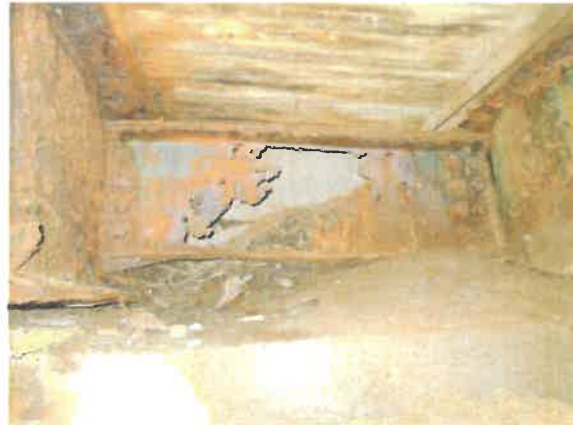
100% Section Loss in Diaphragm
