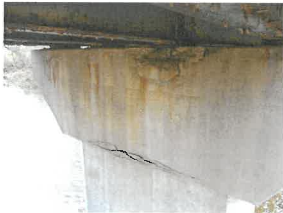
Concrete Spalling at Stringers Bearings
