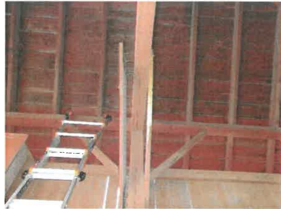
Broken Connection at Crossbeam and Knee Brace
