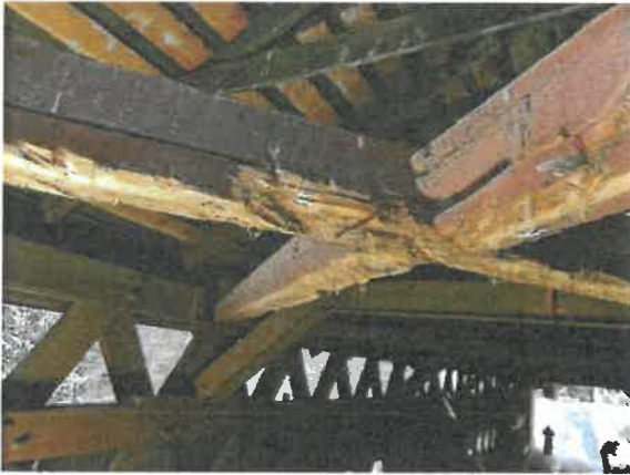
Impact Damage in Diagonal Bracing
