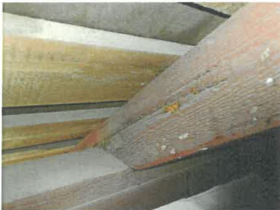
Split in Rafter
