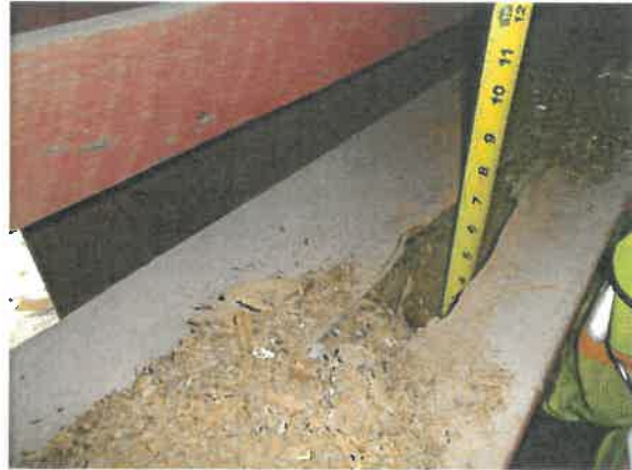
East Truss Top Chord Rot
