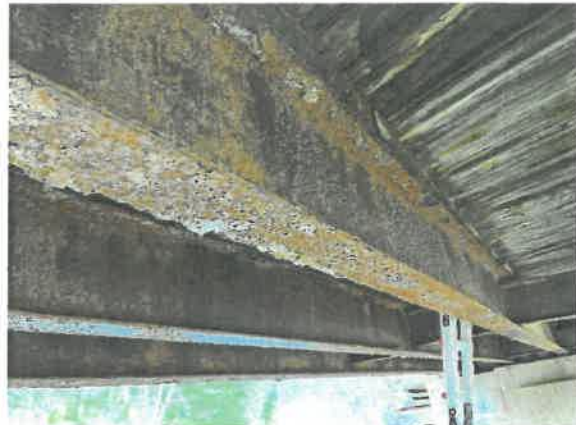
Interior Beam Rusting
