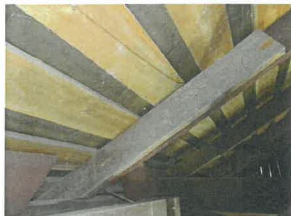
Split in Roofboard and Spliced Rafters
