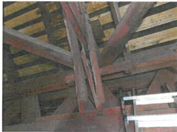
Broken Connection at Crossbeam and Knee Brace
