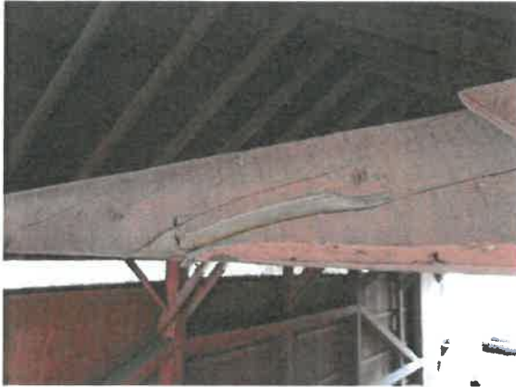
Split in Crossbeam
