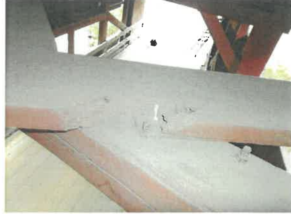
Broken Connection at Cross Beam and Diagonal
