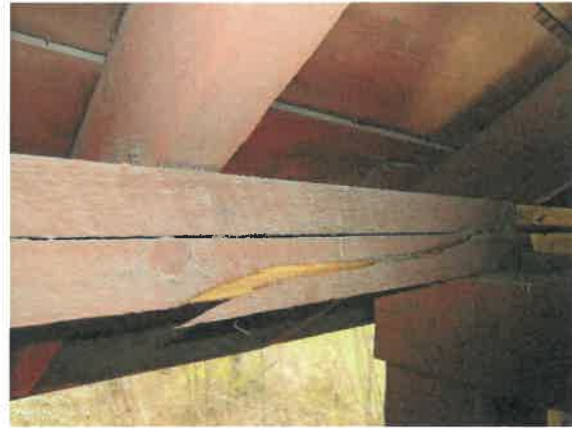
Splits and Breaks in Roof Boards and Rafters
