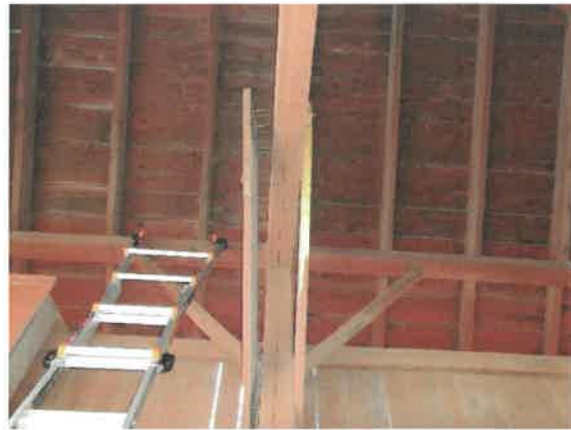
Broken Connection at Crossbeam and Knee Brace
