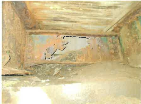
100% Section Loss in Diaphragm
