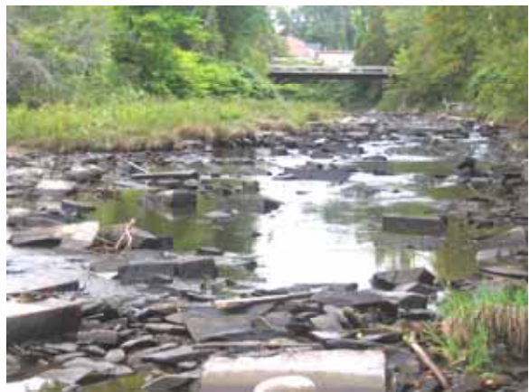
Figure 5.30: Granite tailings in channel downstream of footbridge behind Mobil Station on N. Main Street
