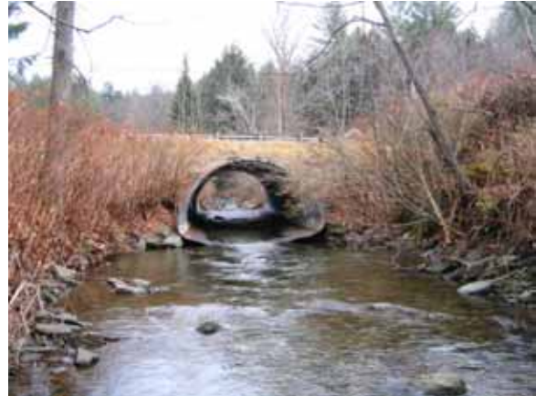
Figure 5.70: Undersized culvert and straightened channel at Route 12A near Little Northfield Road
