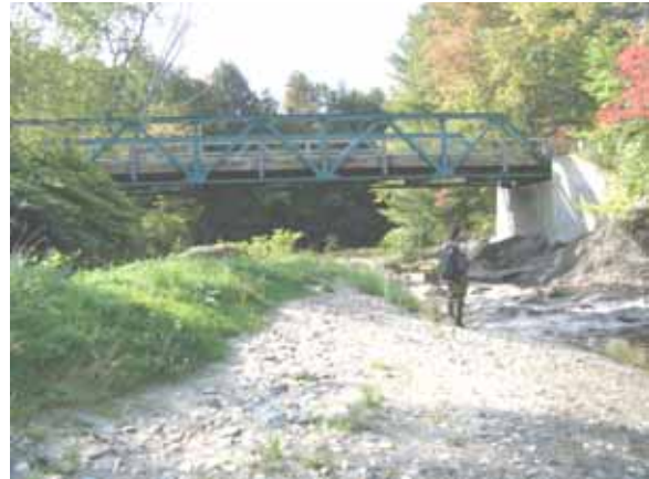
Figure 5.18: Deposition above bedrock constriction near Lovers Lane Bridge
