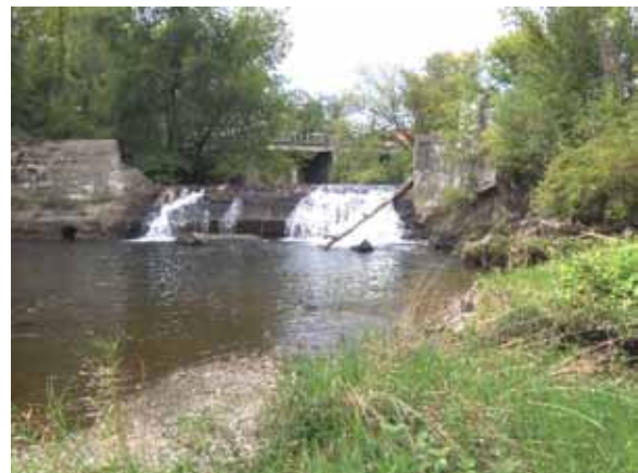
Figure 5.33: Breached dam located downstream of Main Street bridge in downtown Northfield
