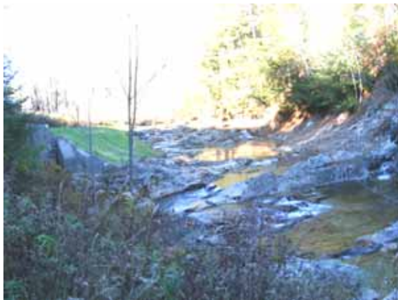
Figure 5.58: Location of removed dam along Cox Brook Road near Pierson Hill with bedrock grade controls and newly planted vegetation
