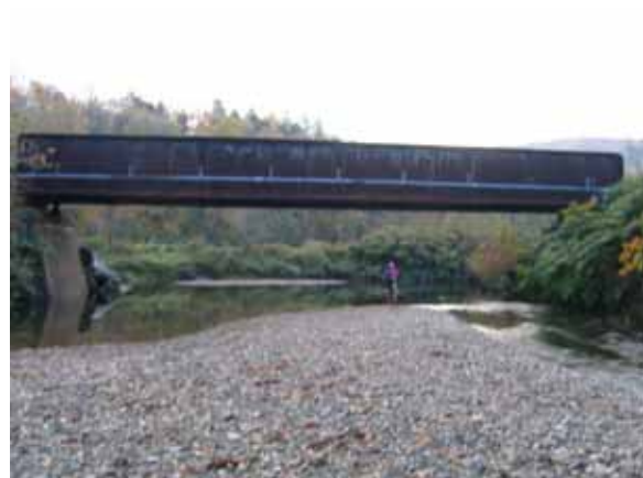
Figure 5.8: Major deposition and planform adjustment downstream of undersized railroad bridge
