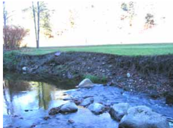
Figure 5.59: Bank erosion along maintained yard with Cox Brook Road in background upstream of second covered bridge on Cox Brook Road
