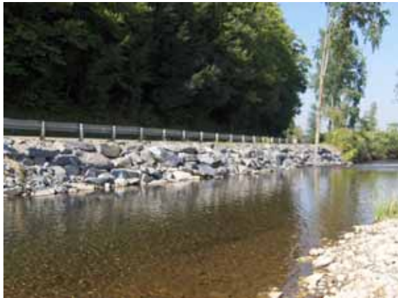
Figure 5.35: Channelized section of Dog River with extensive rip rap and no riparian buffer along Water Street near Norwich University
