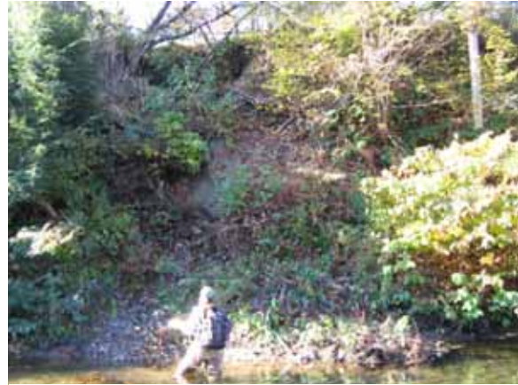
Figure 5.6: Mass failure on right bank near M's RV dealership on Route 12
