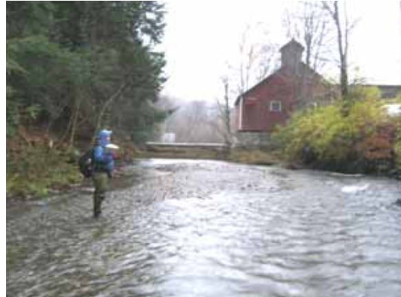
Figure 5.64: Mid channel accumulation upstream of breached dam near the intersection of Route 12 and Lovers Lane
