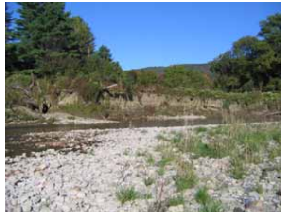
Figure 5.21: Extensive bank erosion on west bank near Berlin-Northfield town line
