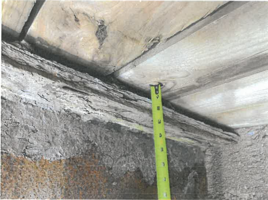
Gap Between Deck & Top of Stringer #4 @ Abutment #1
